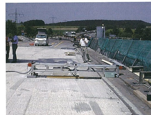
FIGURE 5.24: Portable rail support frame with the magnetizing and sensing carriage during a bridge test (1999).
