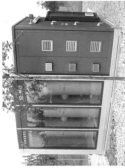
FIGURE 12.40: A resistive SCFCL constructed by Nexans and installed at the Boxberg substation. (Courtesy Nexans-Boxberg.)
