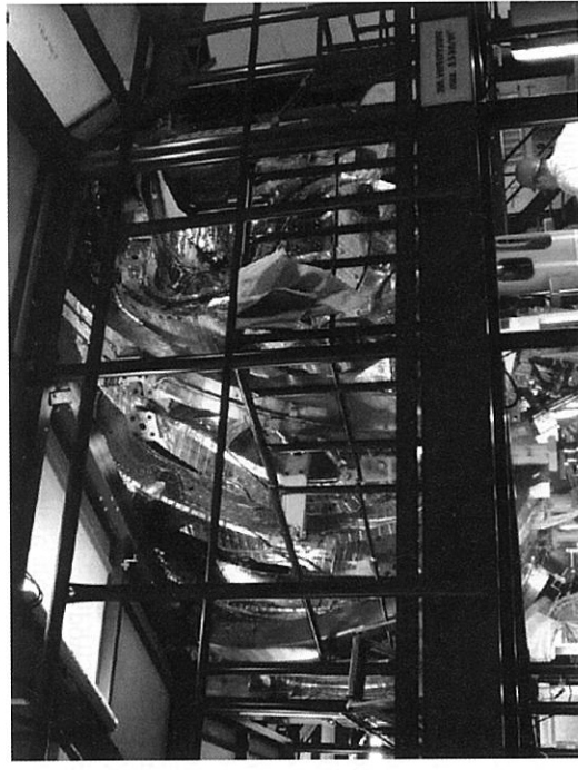
FIGURE 12.37: The W7-X coil system during installation at IPP in Greifswald. (Courtesy of the Max Planck Institute.)
